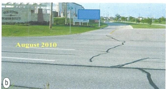
Figure 14. Recent pictures of Hockley fault at Highway 290 Frontage and Fairfield Falls Way roads: (a) taken in April 2010 and (b) taken in August 2010. Note the development of the tiny cracks in (a) into significant cracks in (b).
